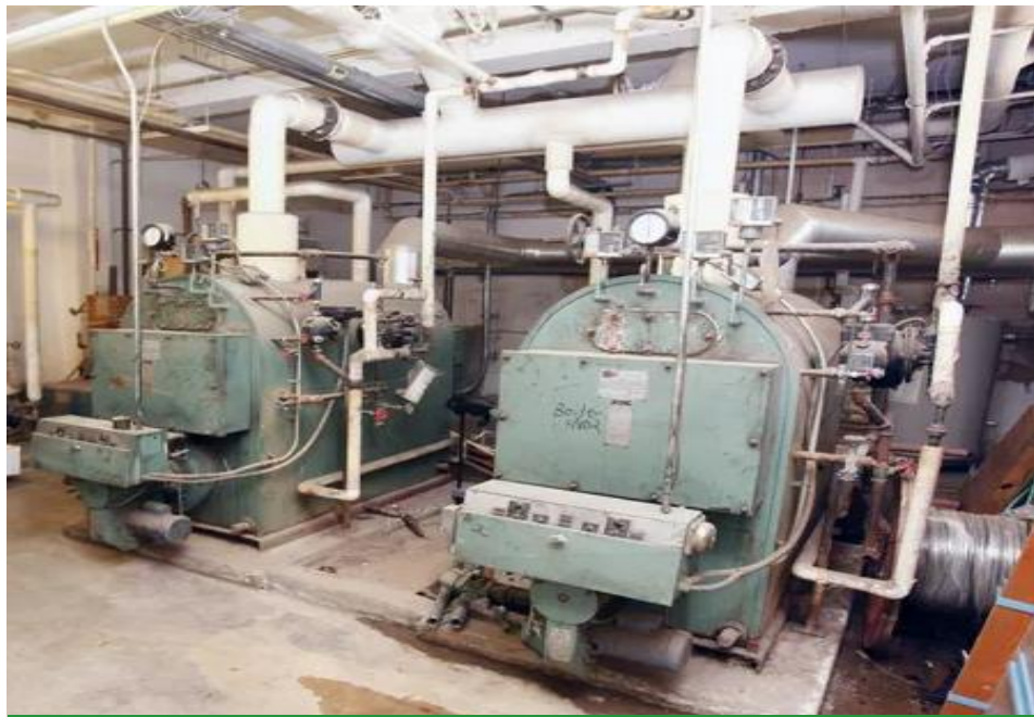
Less Efficient Boiler Systems
